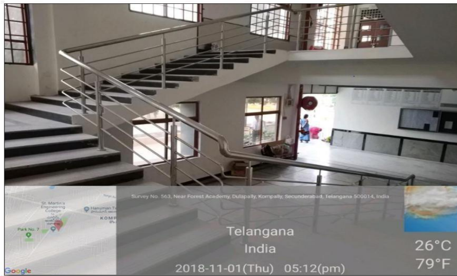
Rail in M.V Block
